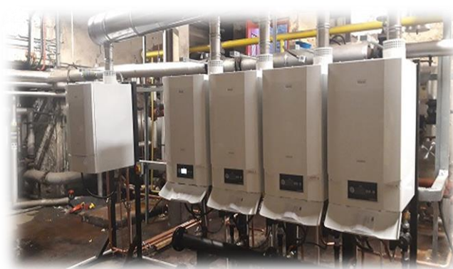
(New eco boilers – West End Campus)
